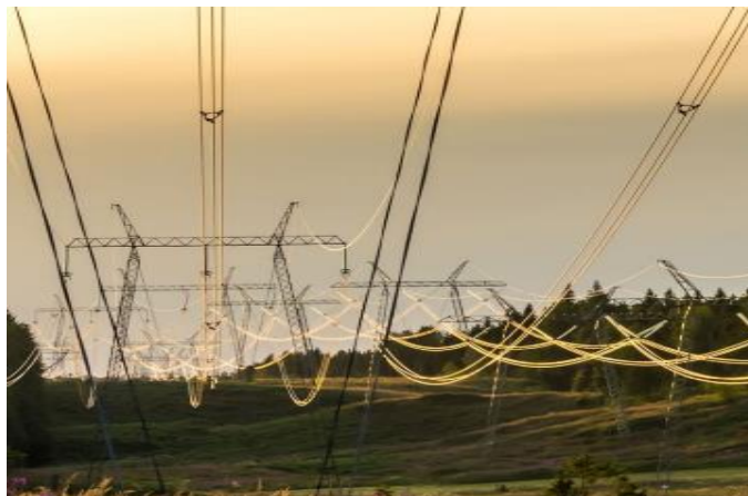
Figure 9. Energy Transmission Towers (source: FINGRID).
